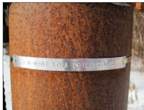
A Protected Wellhead with identification banding
