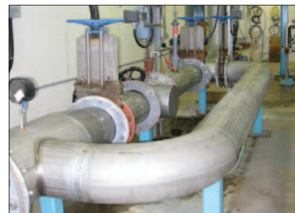
Drinking water distribution piping
