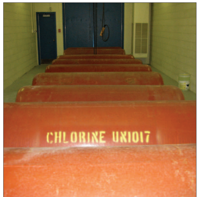
Chlorine gas tonners, Exploits Regional water treatment plant
