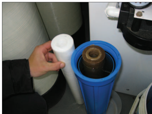
Filters for the treatment of drinking water
