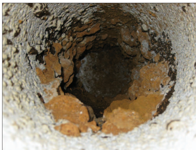
Scaling on the inside of drinking water distribution piping
